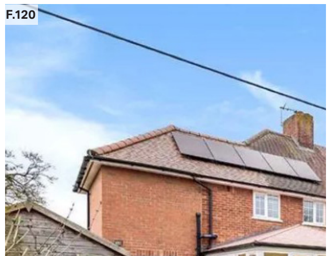
Figure 120: Solar panels installed on the south-facing pane of the roof of existing house in Wetheringsett. (Source: onthemarket.com)
